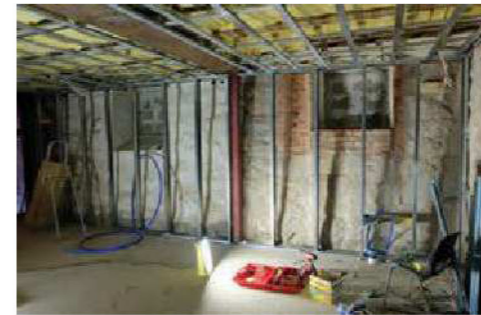
■ About 3,000 meters of Cat 7 cables were used to snake around brick walls
